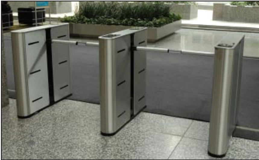
Turnstiles in the lobby can slow a visitor, thus giving security more time to view passes and request a valid identification or access card. This one comes from Smarter Security Solutions, Inc.
